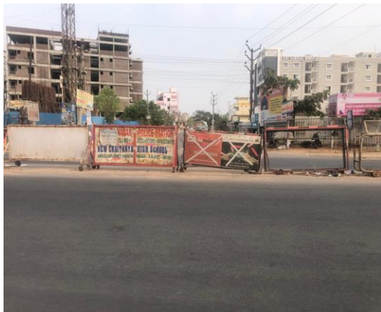
Fig.11: At chainage 2.600 Km, Barricades provided are damaged. Need to be replaced.
