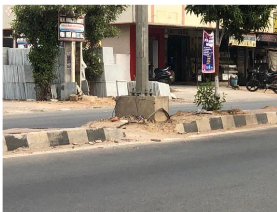
Fig.12: At chainage 3.000 Km, Unauthorised opening in the median for illegal movement of two wheelers leading to unsafety.
