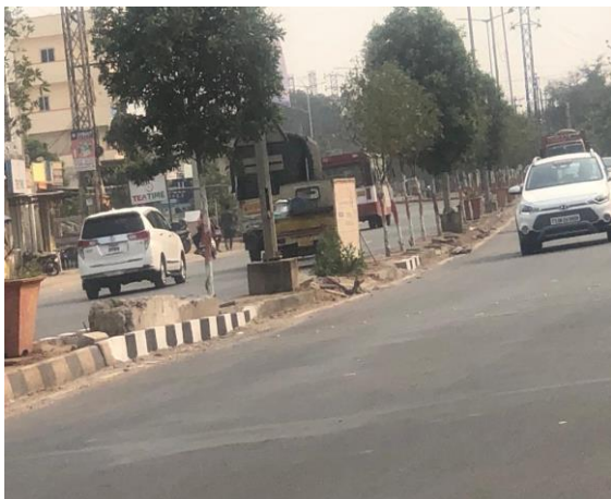
Fig.6: At chainage 1.300Km, Median is damaged as shown in figure.
