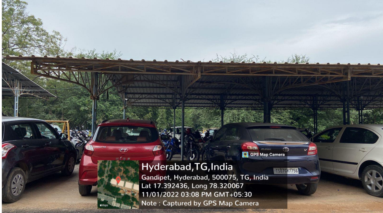
CC TV cameras are installed at the parking
