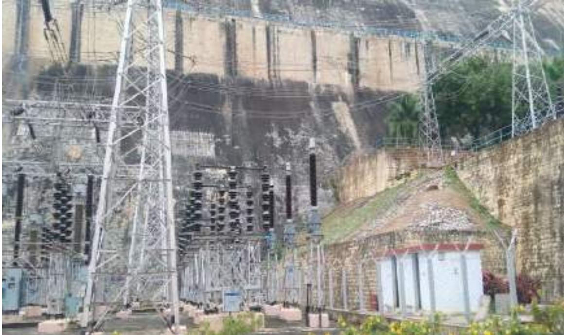
Bus bar system
