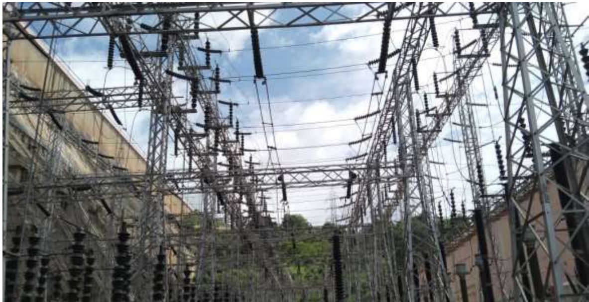
Bus bar system
