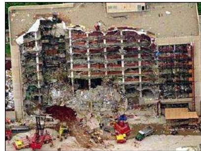
Figure 1 – Progressive Collapse of Building
